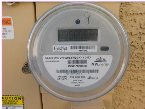
ELECTRICAL SERVICE Electric Meter Location
