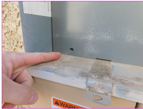
SERVICE PANEL Dead Front Cover Condition
