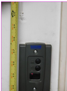
OVERHEAD GARAGE DOOR Automatic Opener Switch
