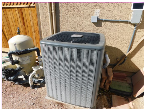
CENTRAL AIR CONDITIONER General Condition
