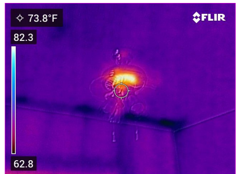
THERMAL IMAGING Electrical
