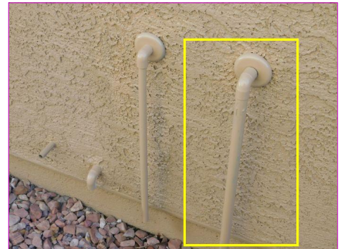
WATER HEATER TPR Discharge Pipe
