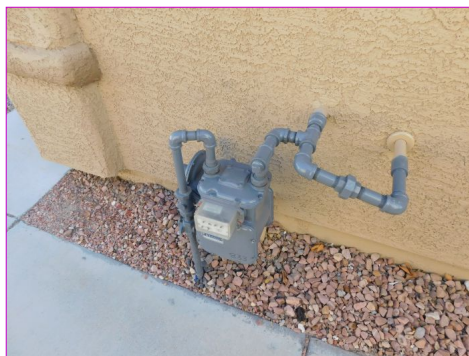
GAS SYSTEM Main Gas Shut-off
