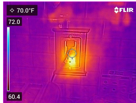
THERMAL IMAGING Electrical
