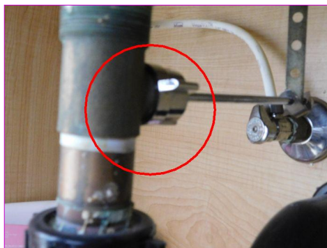
UPSTAIRS HALL BATHROOM Undersink Plumbing
