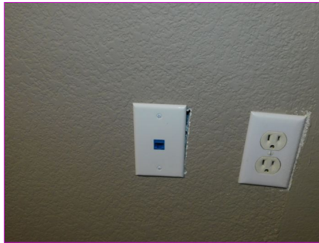
2nd UPSTAIRS BEDROOM Electrical Receptacles
