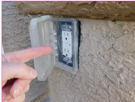
EXTERIOR ELECTRICAL Exterior Electrical Receptacles
