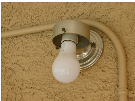
EXTERIOR ELECTRICAL Exterior Lighting
