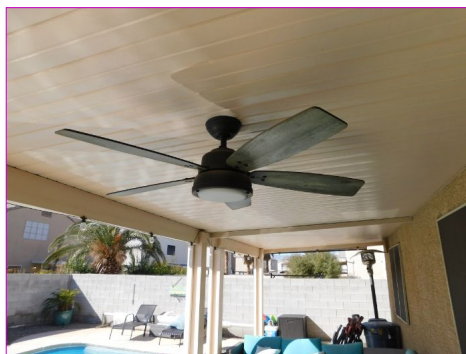
EXTERIOR ELECTRICAL Exterior Lighting
