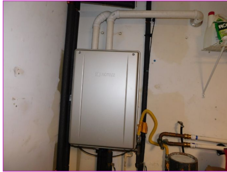
WATER HEATER Water Heater Type
