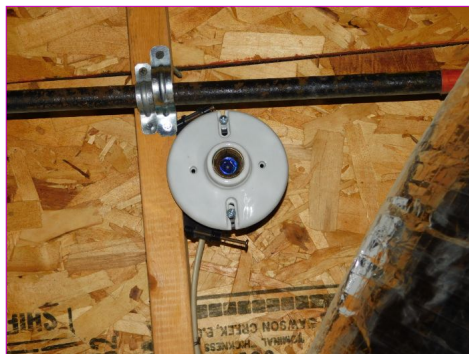
ATTIC Attic Electrical
