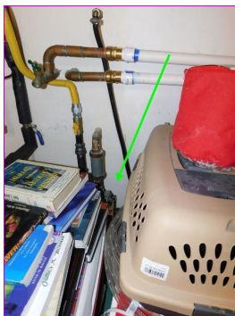
WATER SUPPLY PIPES Main Water Shut-off
