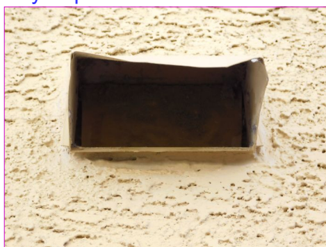
LAUNDRY ROOM Dryer Venting
