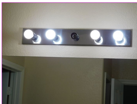
MASTER BATHROOM Light Fixtures
