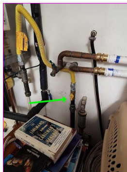
WATER HEATER Fuel Supply
