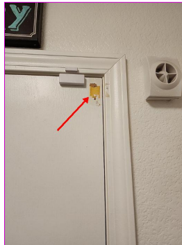
LAUNDRY ROOM Exterior Door Condition
