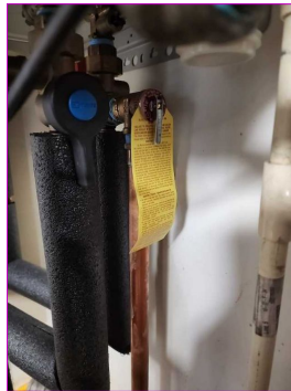
WATER HEATER Pressure Relief Valve
